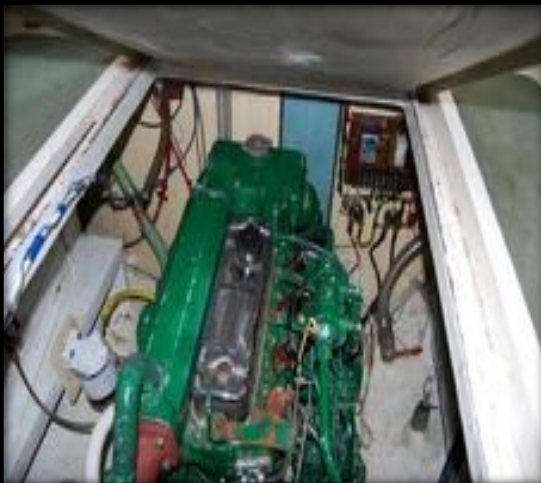
Typical Thornycroft engine bay
