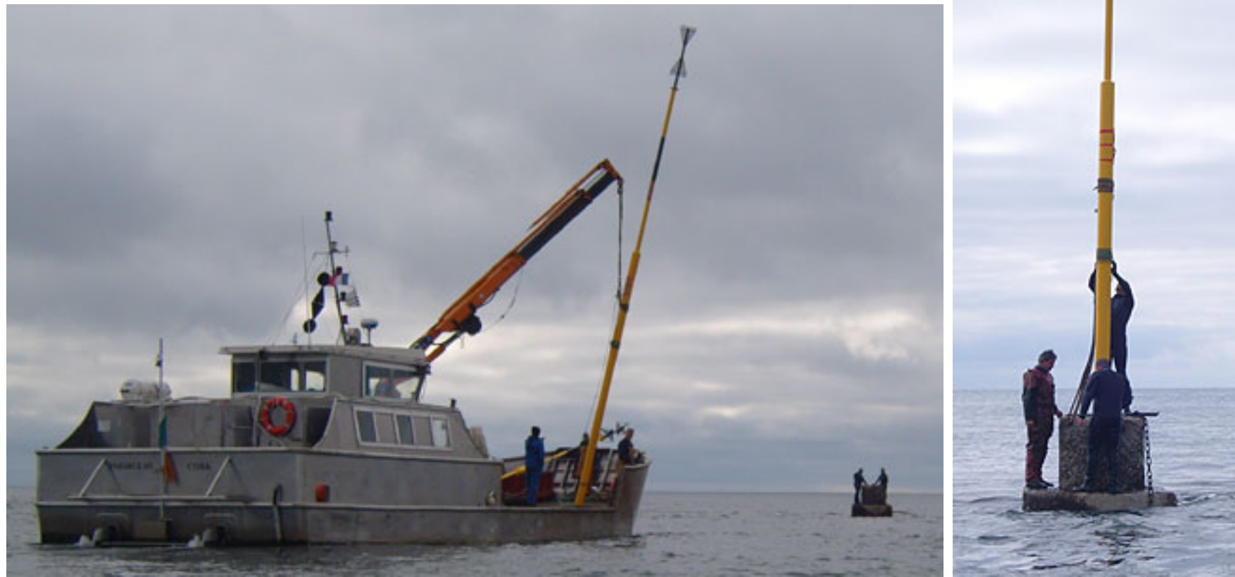
Assistance Phares & Balises : pose de la balise renforcée du "Trehou" à Groix : diam 160 - 1,6 tonne. Assistance to the Lighthouses department, in very shallow waters.
