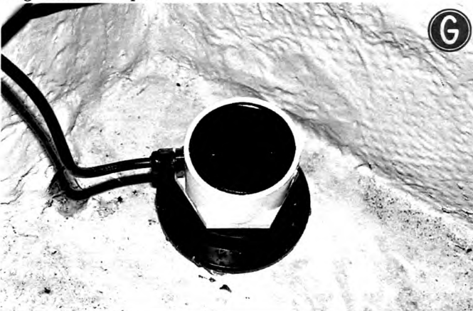
G: Once set (24 hours +), the transducer assembly is screwed into position with a good big dollop of Fix-A-Tap lubricant on the face. But before doing so, wind it anti-clockwise a number of turns.
